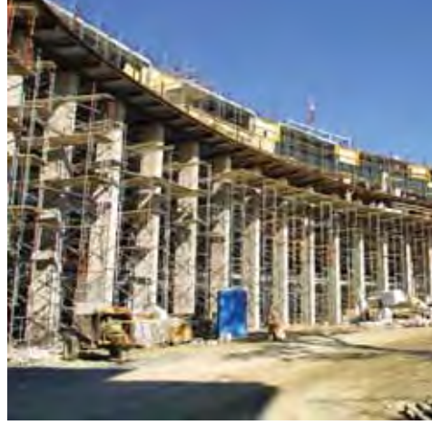
The first phase of Olin campus construction took place from early 2000 through 2005.
